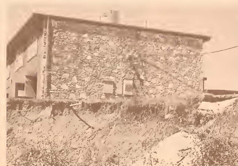
Unprotected soil near this apartment building washed away during heavy rains. The concrete waterway (right) has been damaged and the service pipes (left) are exposed.
